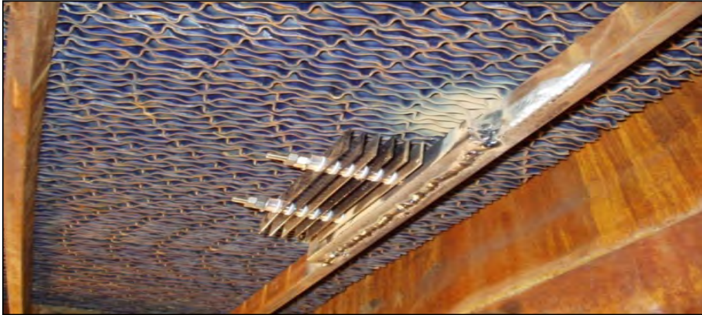
Field coupon racks installed on rotating air heater baskets at 20 units
